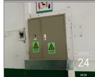
Photo of fire safety equipment Electricity box label.jpg
