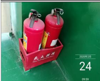
Photo of fire safety equipment Fire extinguishers.jpg
