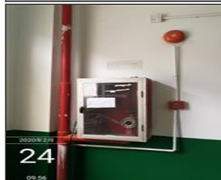
Photo of fire safety equipment Fire hydrant and fire alarm.jpg
