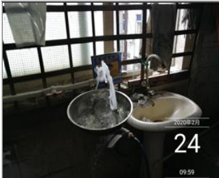
Photo first aid facilities Eye washing facility.jpg
